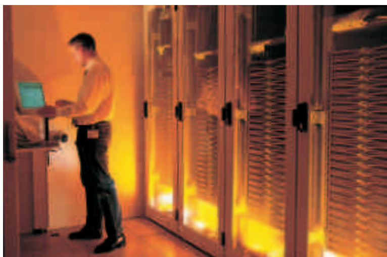
Hardware expert Felix Uellendahl in the server room of the Bayer Pharmaceutical Research Center with the Linux machines in water-cooled cabinets.
